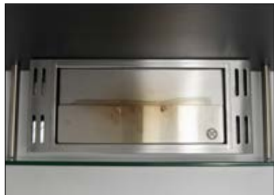
The steel plate now covers the opening and thus smothering the fire
